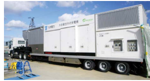
Large-Capacity Air-Cooled Generator
