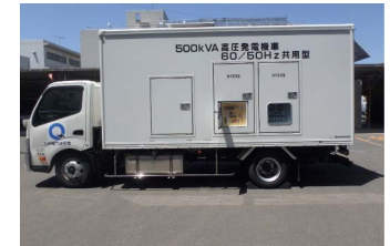
High-voltage generator truck
