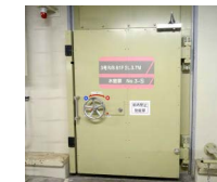
Overflow countermeasures (watertight door)
